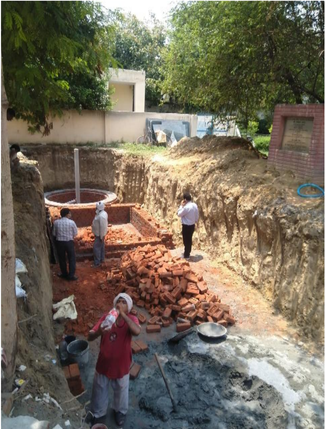
Construction of Structures for Co-solving of Water Logging and Ground Water Depletion Issues in Officer's Colony, Sector 15A of Faridabad City of Haryana State of India
