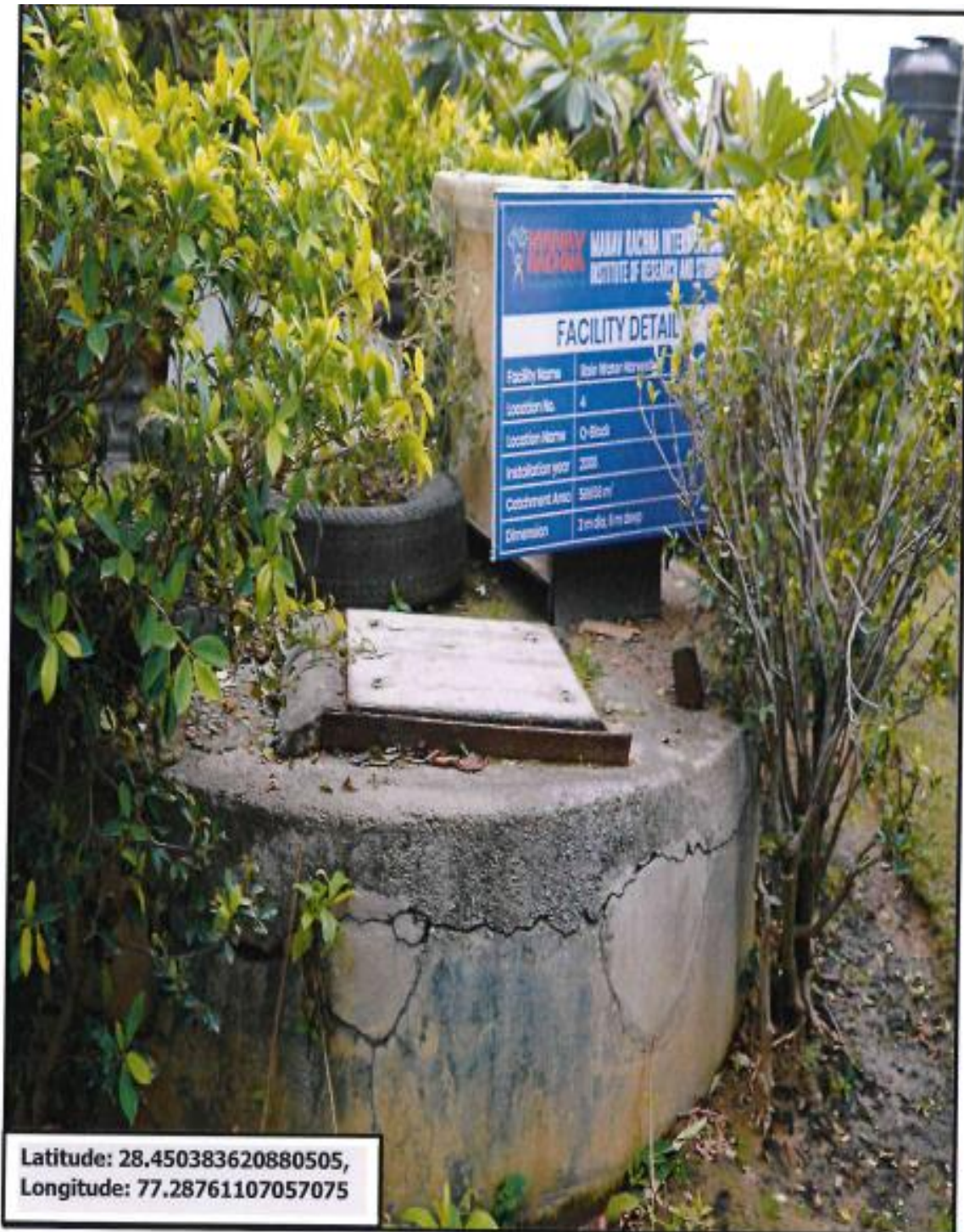
Rain Water Harvesting Q Block
