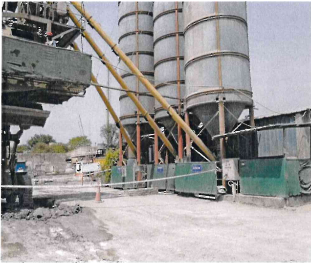
Cement and fly ash silos
