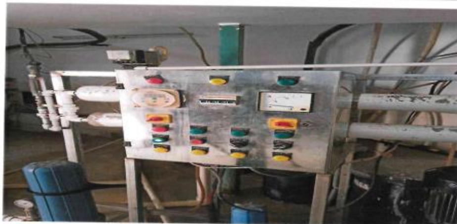
RO system installed in the Campus
