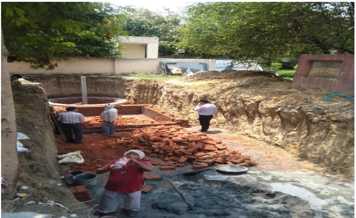
Construction of Structures for Co-solving of Water Logging and Ground Water Depletion Issues in Officer's Colony, Sector 15A of Faridabad City of Haryana State of India
