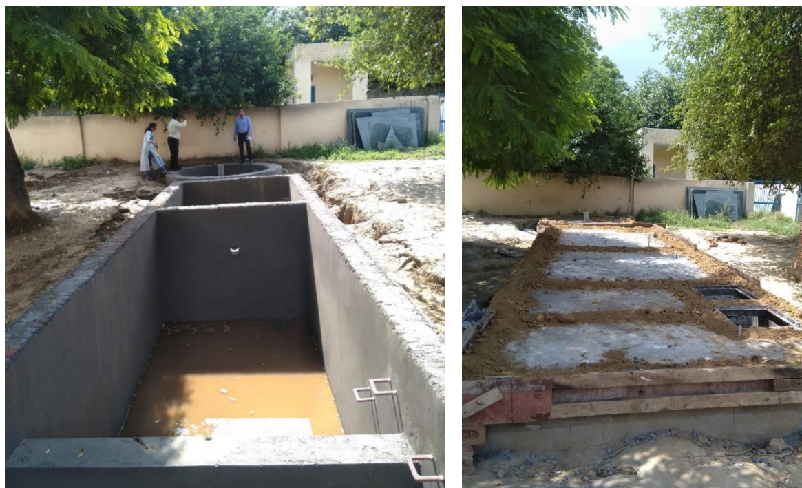
Fig 10. Photographs of constructed desilting and coagulation chambers and dug cum recharge well at Officers Colony.
