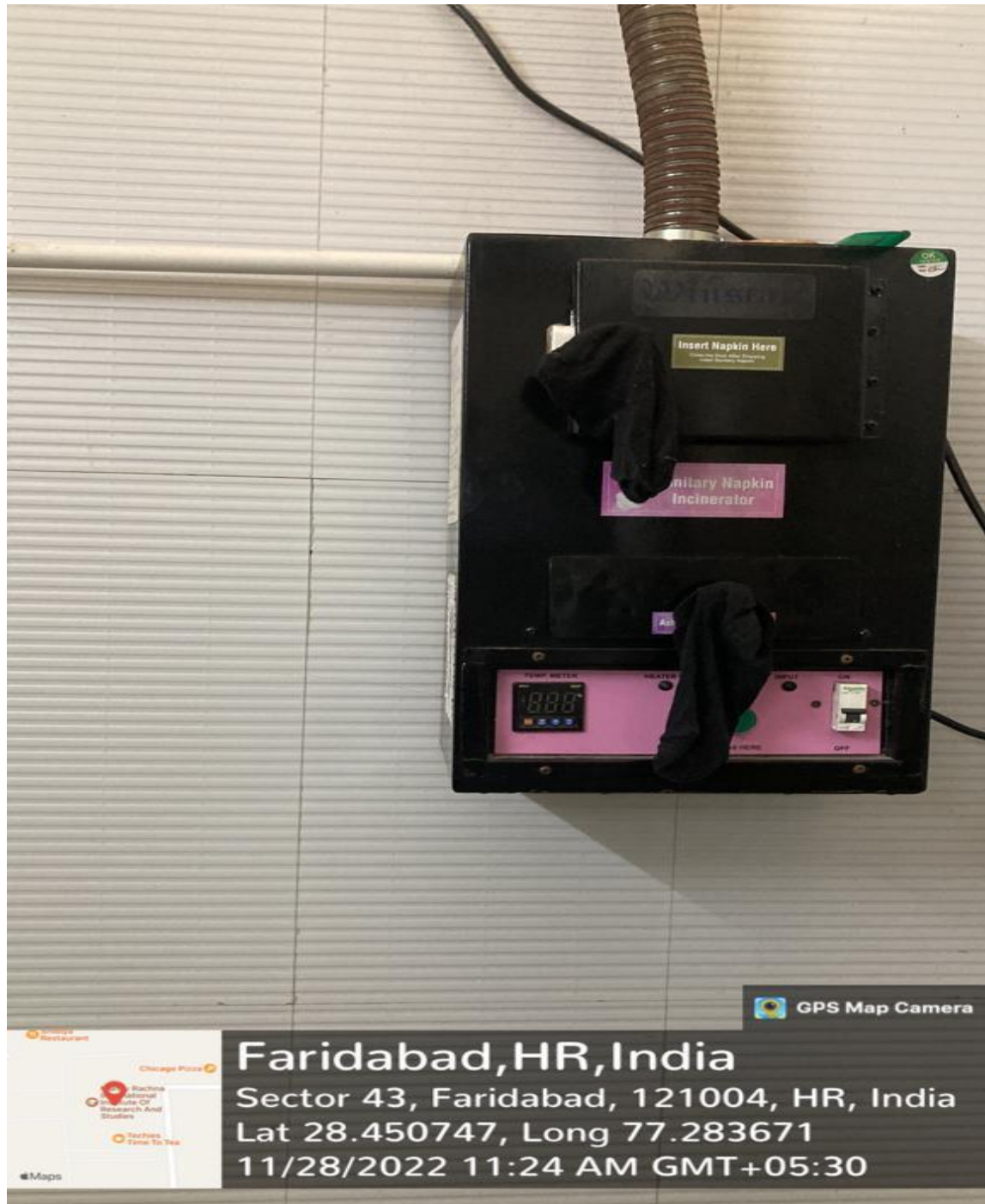
Sanitary Pad incinerator
