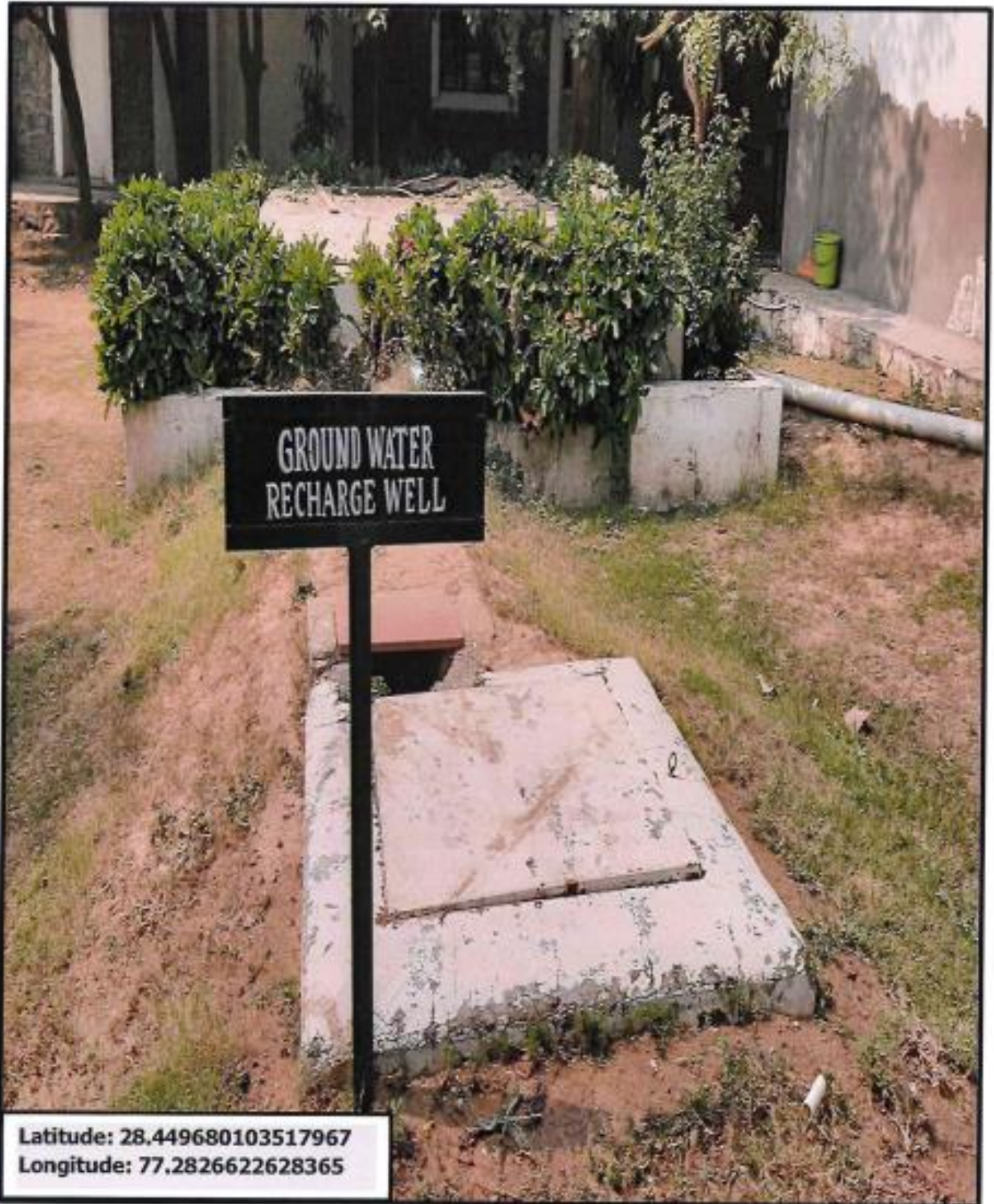
Rain Water Harvesting Ground Water Recharge Well C Block
