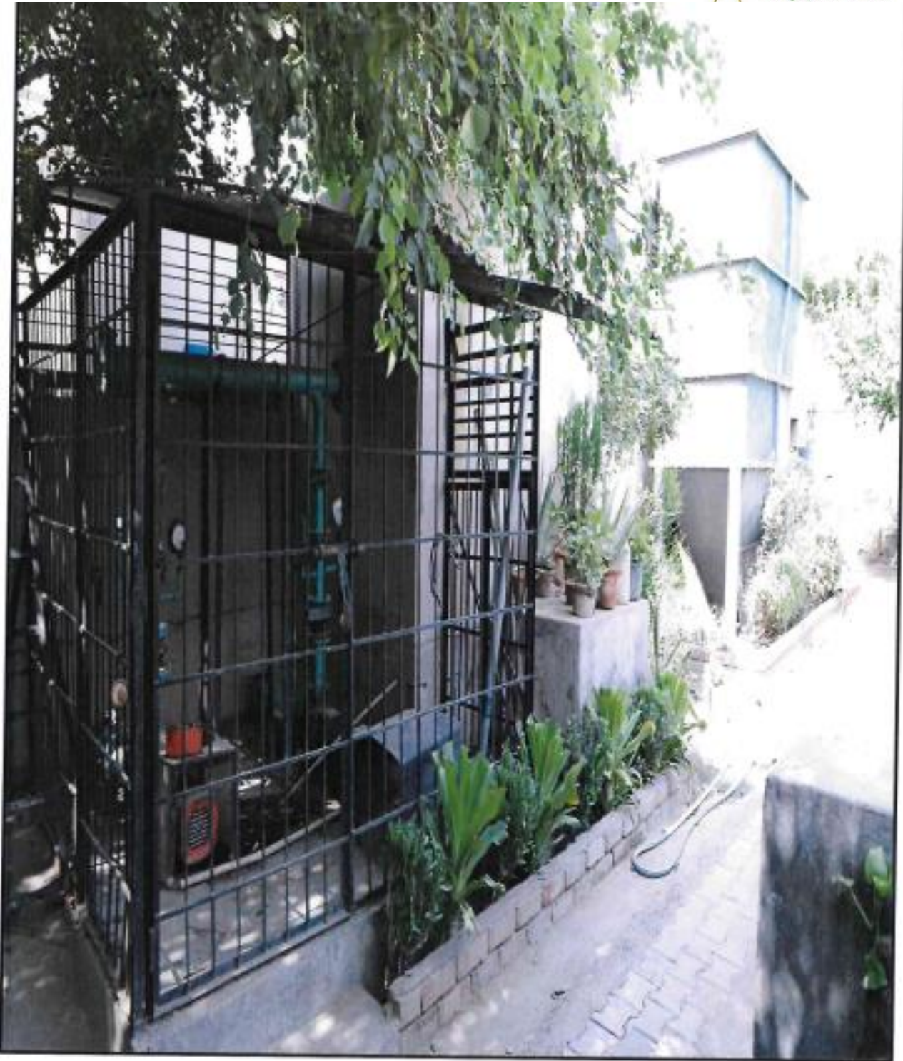
Treated Water Distribution, Sewage Treatment Plant
