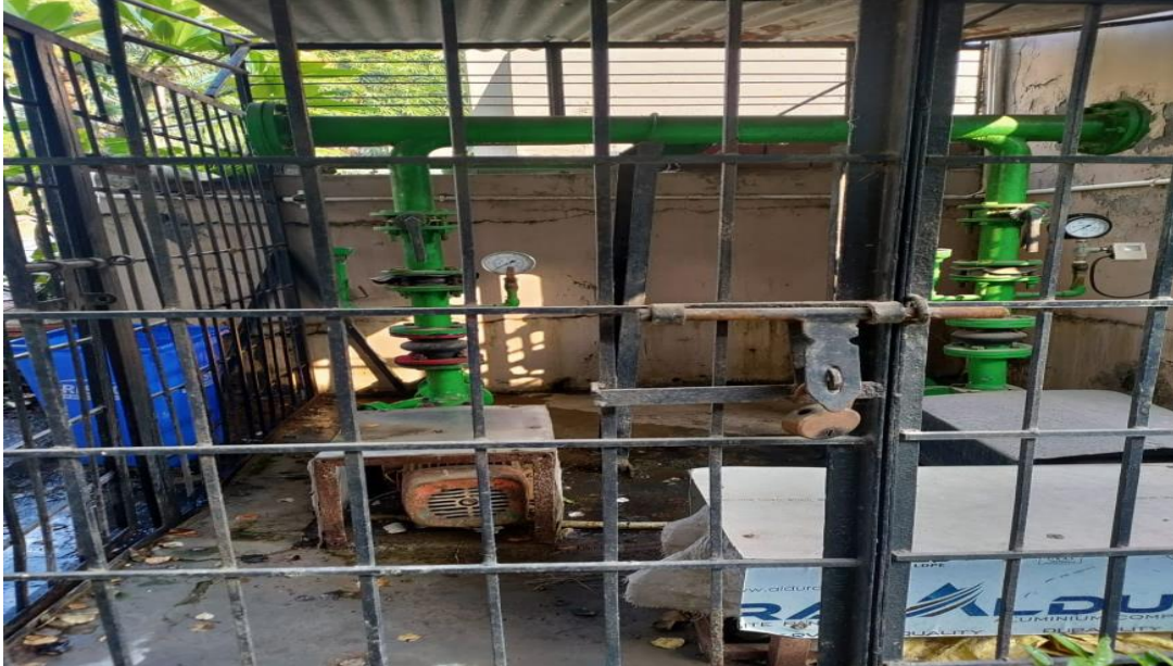
Pumping system of clean water
