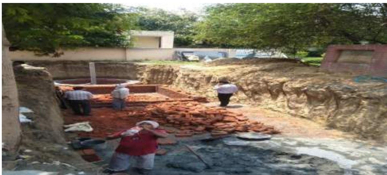
Construction of Structures for Co-solving of Water Logging and Ground Water Depletion Issues in Officer's Colony, Sector 15A of Faridabad City of Haryana State of India
