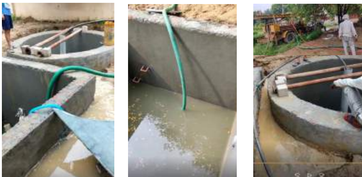
Fig 11. Photograph showing slug testing arrangements at Officers colony, Faridabad
