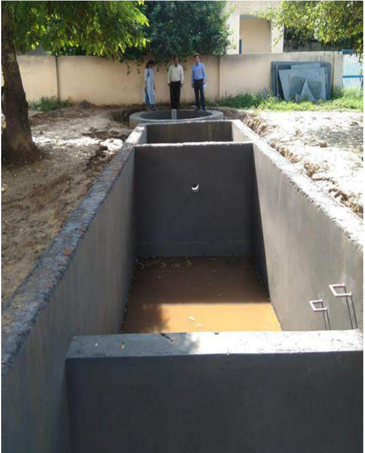
Constructed Structure at Officer's Colony, Sector 15A of Faridabad City of Haryana State of India
