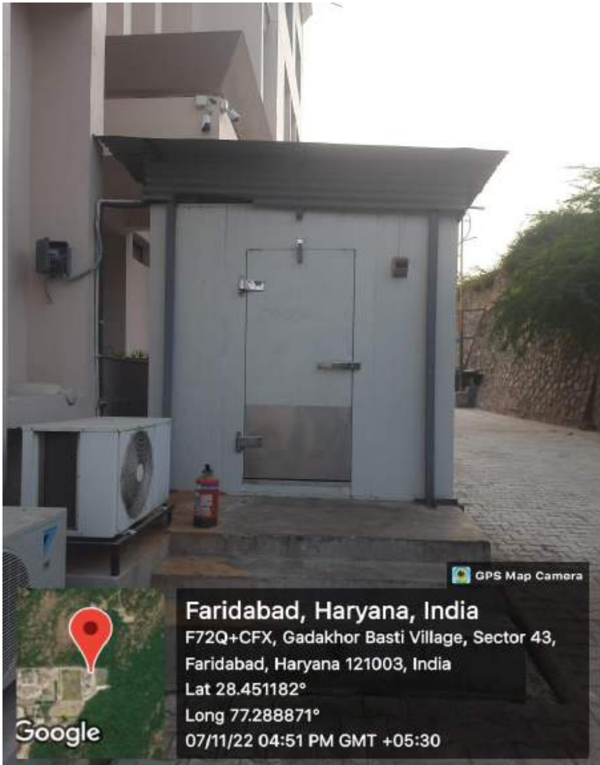
COLD STORAGE ROOM 27 FOR FOOD WASTAGE (Walk-in to keep all food wastage at correct temp for future Process)
