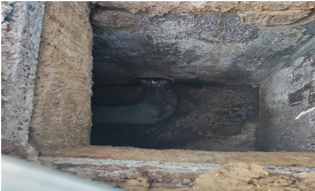
Inlet of sewage water into STP
