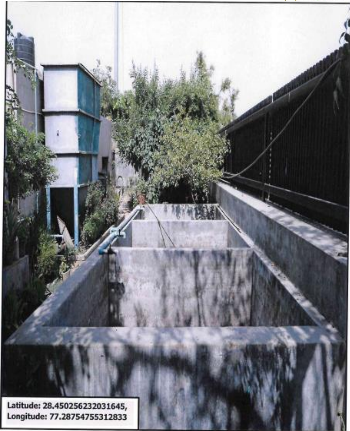
Sludge Dry Bed Sewage Treatment Plant Alternate View
