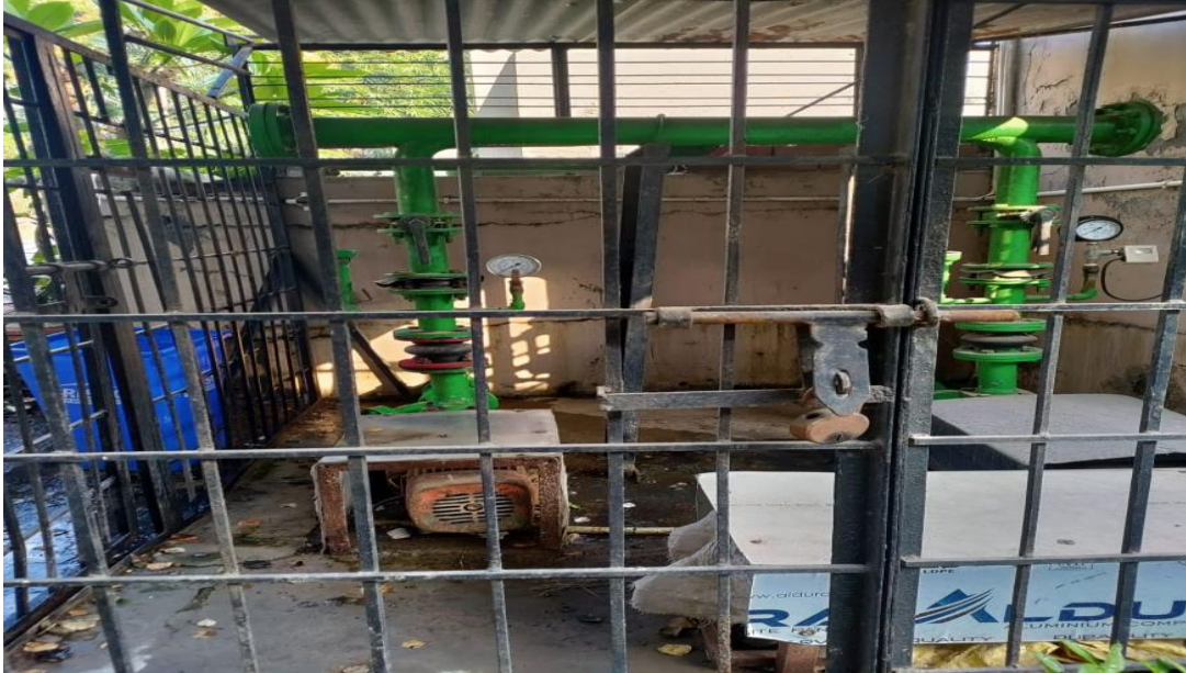
Pumping system of clean water
