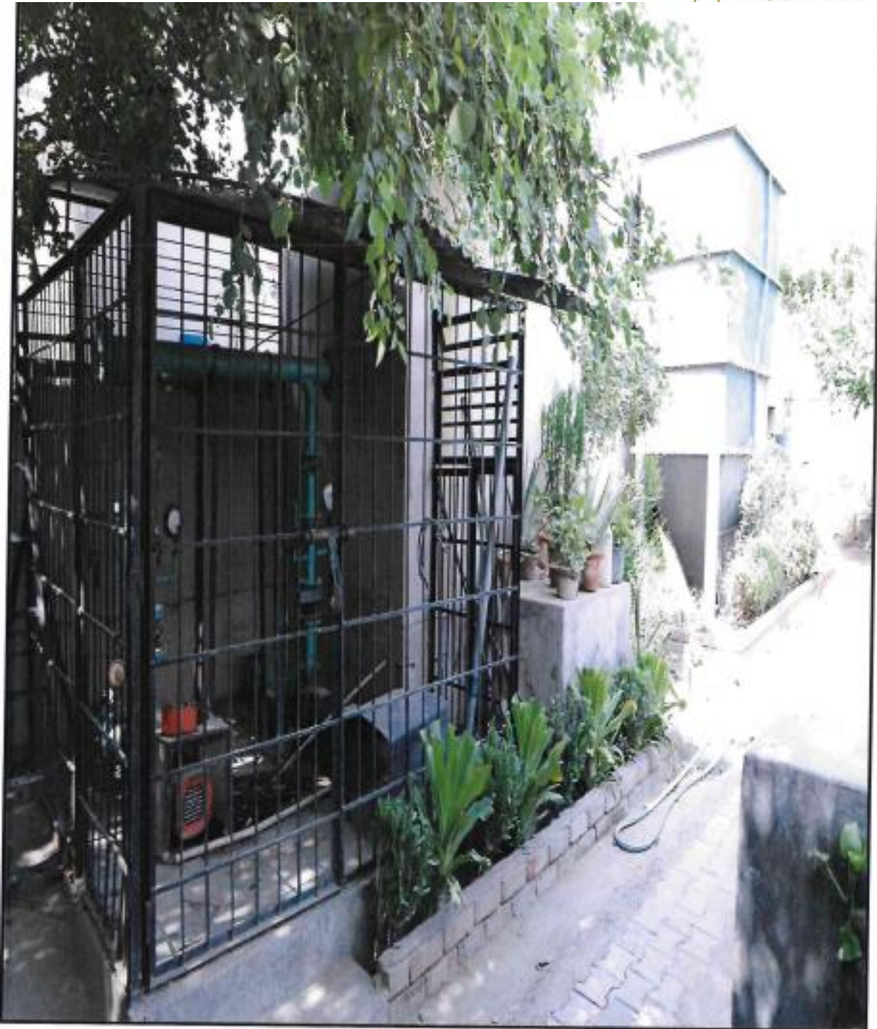
Treated Water Distribution, Sewage Treatment Plant
