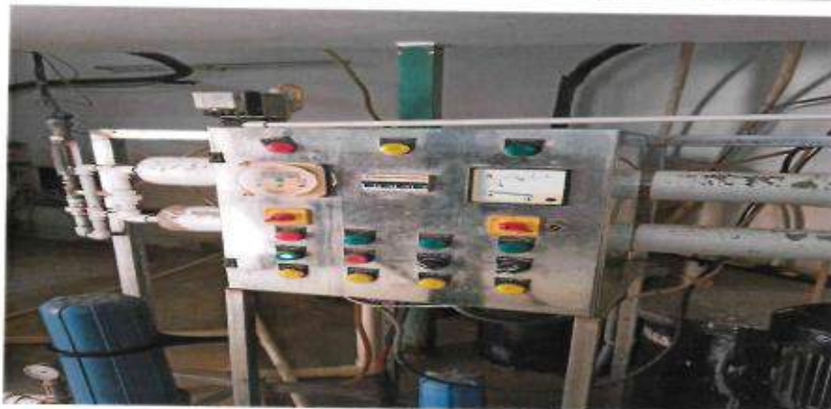
RO system installed in the Campus
