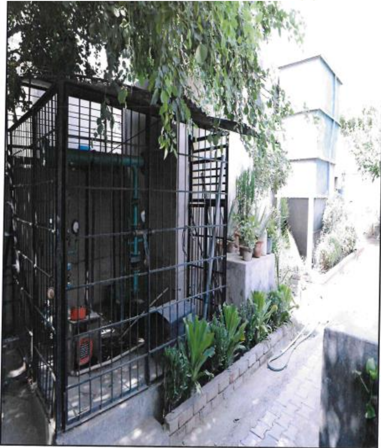
Treated Water Distribution, Sewage Treatment Plant
