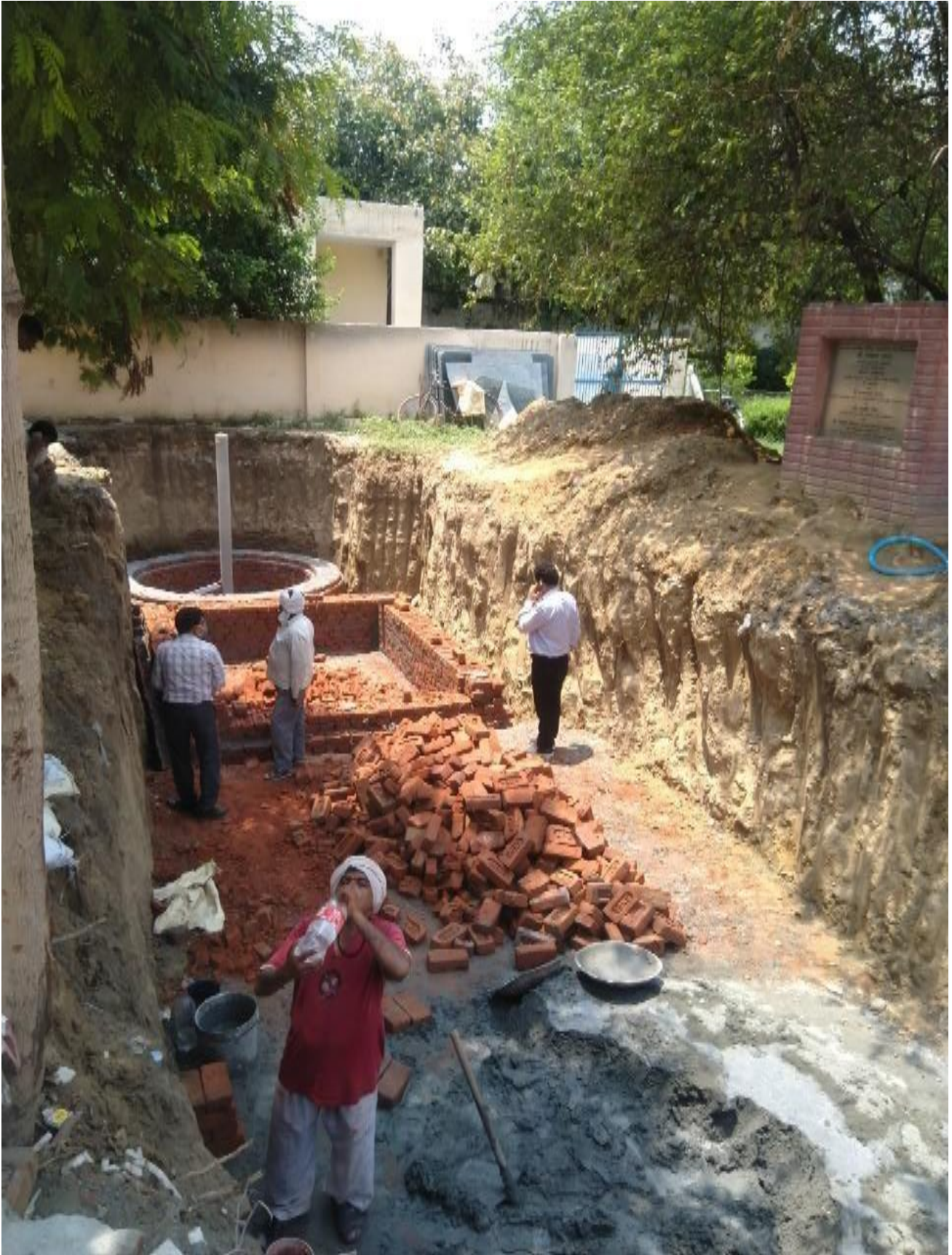
Construction of Structures for Co-solving of Water Logging and Ground Water Depletion Issues in Officer's Colony, Sector 15A of Faridabad City of Haryana State of India
