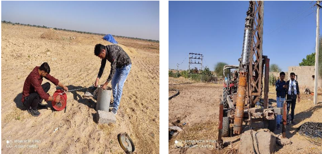
Fig 10.2: Measurement of open tube well depth by water level meter and visit of a new construction site of tube well
