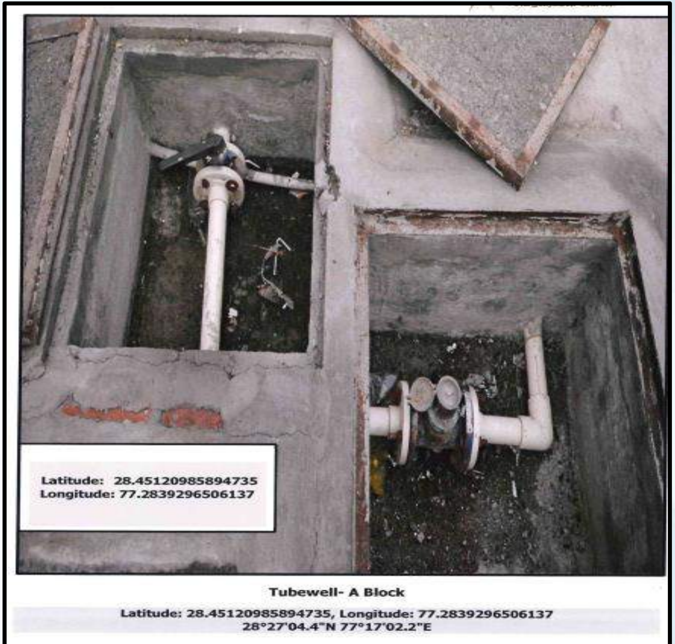
Tubewell-1: Location- A Block
